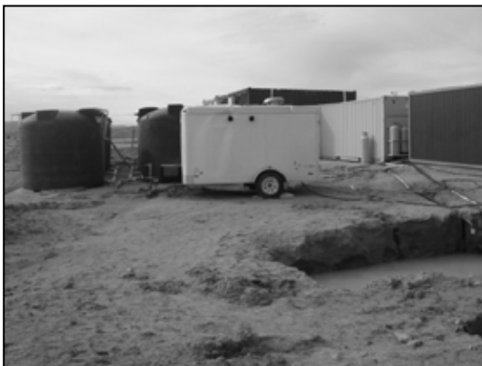
Figure 43. Typical shower units with pump station and water storage units.
